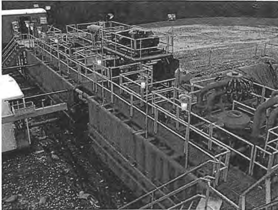
Photo 5.16 - Drilling rig mud system (blue tanks)
